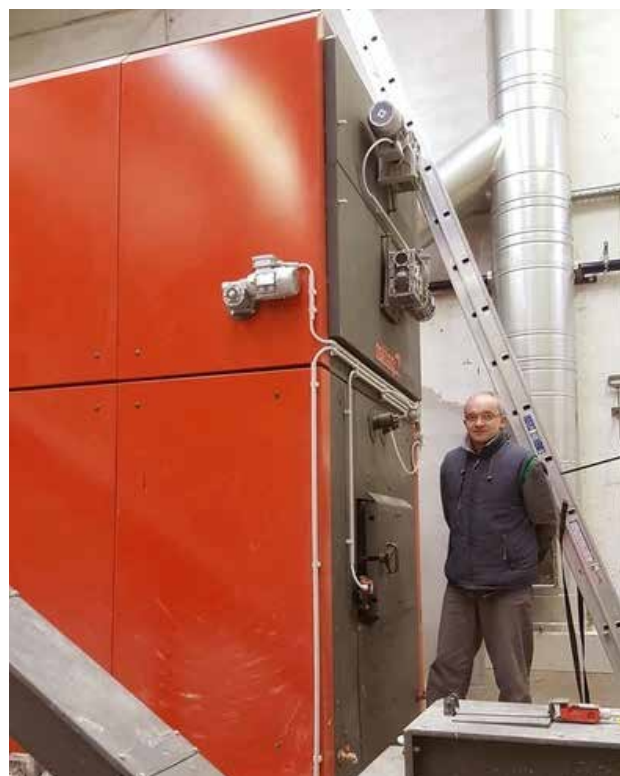
□ Kotao na biomasu Nolting LCS-RU 1150/1300 kW u AKRIPOL-u, Trebnje, Slovenija
